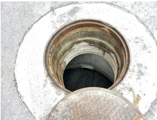
Figure 1: May 17, 2019 sediment in splitter vault up to the input pipe.
