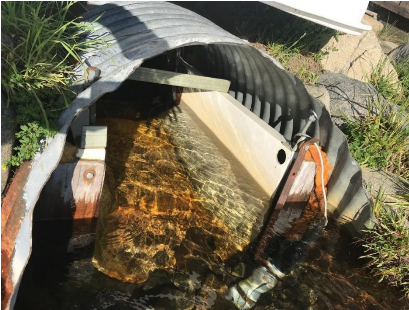
Figure 121 Backwatered conditions at the Tahoma catchment outfall due to high lake levels, July 17, 2019. Lake water extends into the flume.
