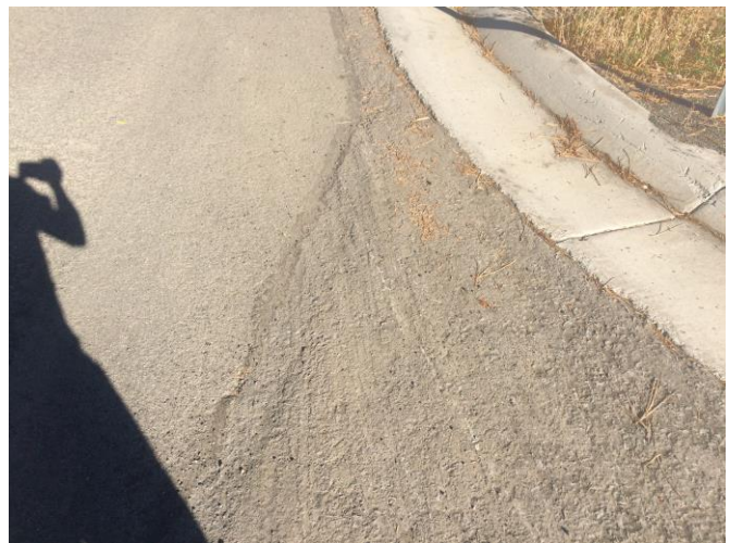
Figure 4: November 1, 2017 sediment on pullout.
