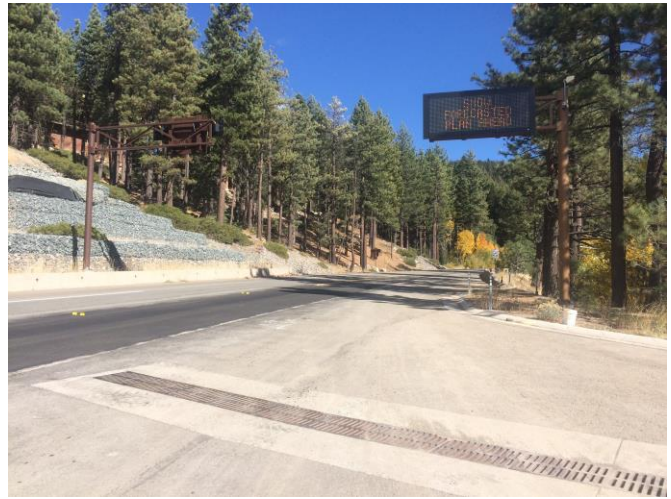
Figure 2: October 19, 2017 sediment on pullout and road.
