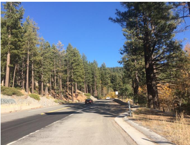
Figure 3: November 1, 2017 sediment on pullout and road.
