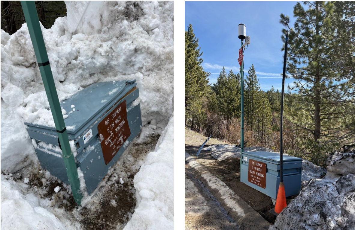
Figure 1 Damage to equipment box and meteorological station pole tilted backwards on February 25, 2026 (left) and box and pole righted to correct position March 17, 2026 (right).
