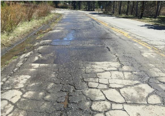
Figure 2 Elks Club Drive prior to repaving. (R Wigart)
