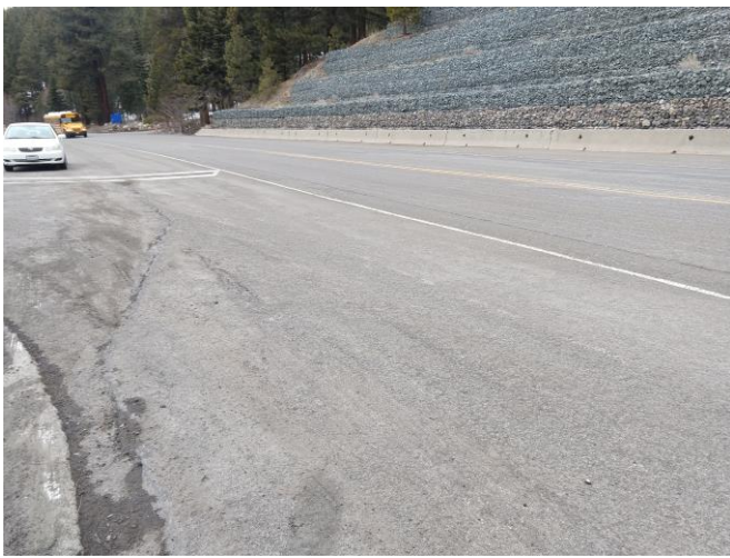
Figure 3 Pullout on SR431 on January 27, 2022.
