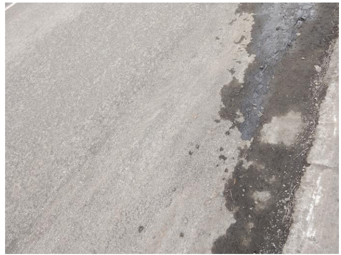
Figure 2 Sediment accumulation on SR431 on January 27, 2022.
